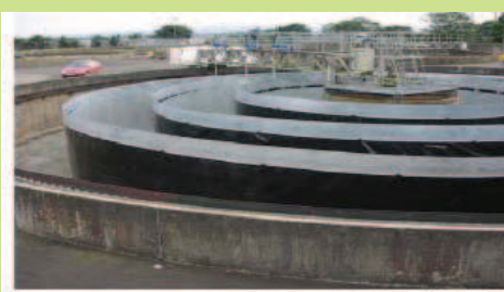
ABR installation at Culmore WWTW, Northern Ireland
